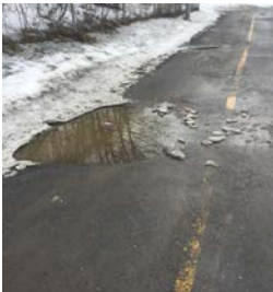
Water covered dip in pathway to South Keys Transit Station
